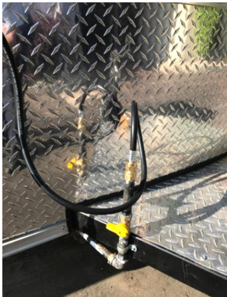
Fuel Line Shutoff w/ 1/4 turn valve
