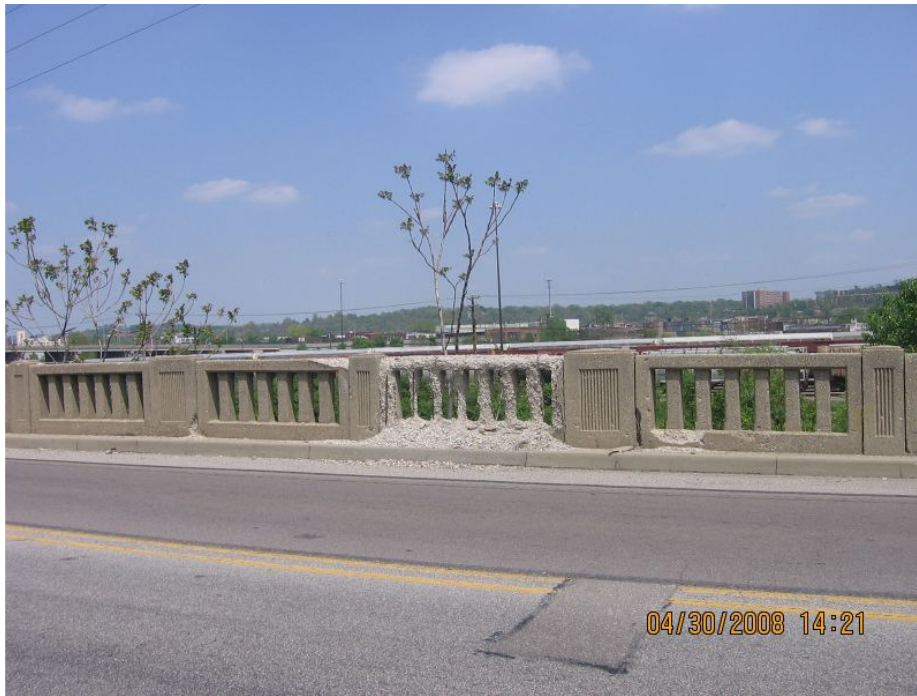
Disintegration of railing exposing steel reinforcement most likely due to salt spray.
