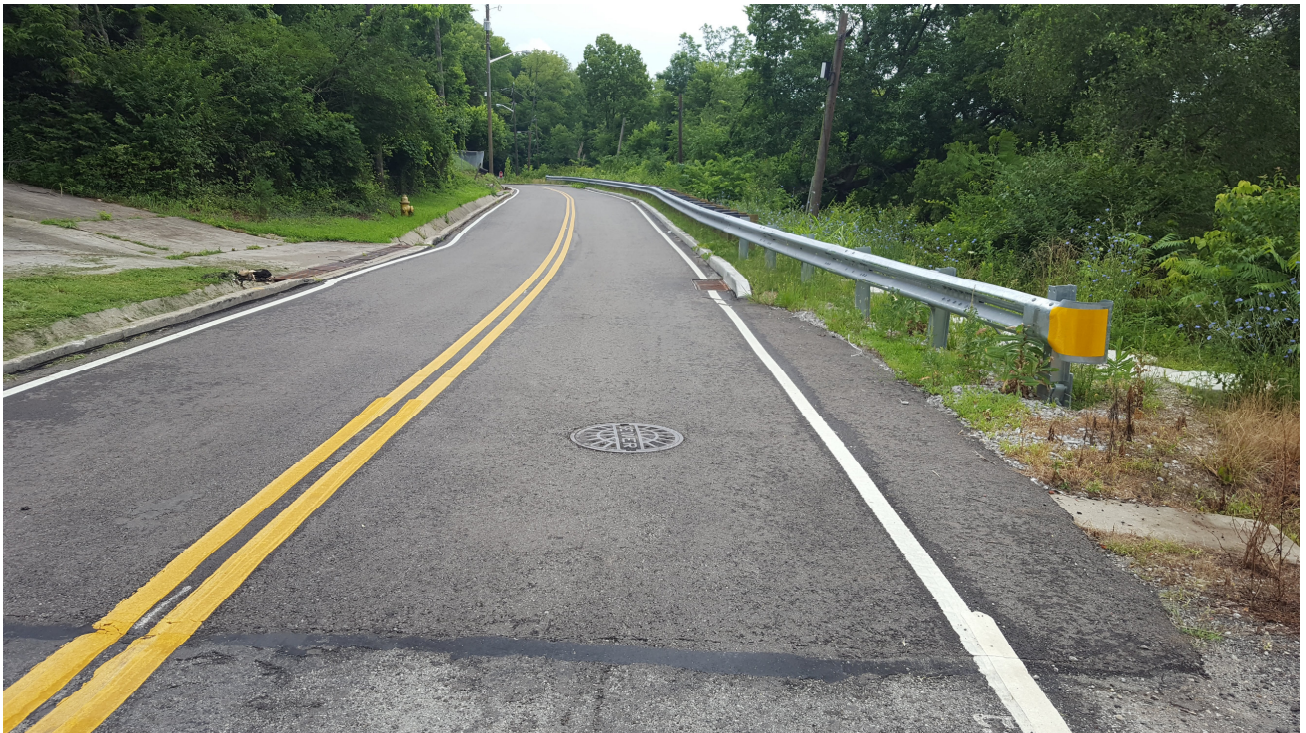
Newly paved surface of Hillside Avenue looking east towards Tyler Street. Roadway stabilized with a drilled pier retaining on the downhill side of the guardrail.
