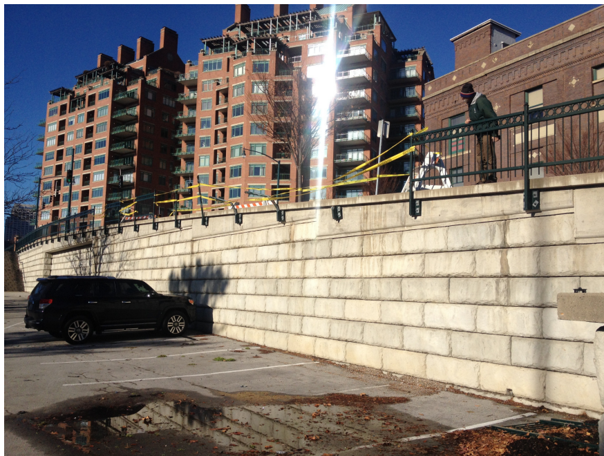
Seventy-two feet of railing needed to be replaced on the Riverside Drive Retaining Wall (Wall #335-143B) due to an automobile accident on December 27, 2016.
