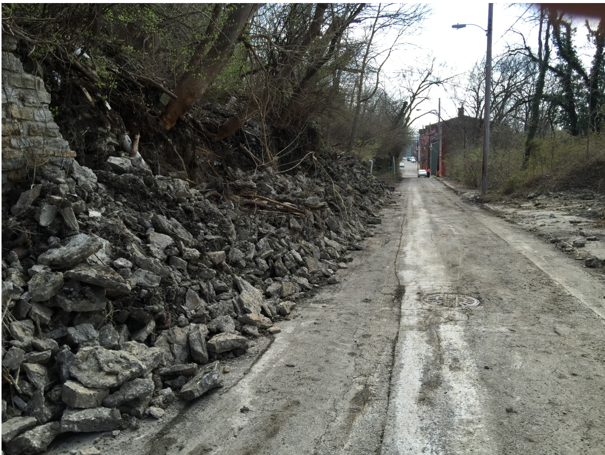
Looking east down Peete Street. Public Services cleared the retaining wall debris from the roadway and stockpiled the stone against the slope to support it. Photo taken on March 3, 2016.
