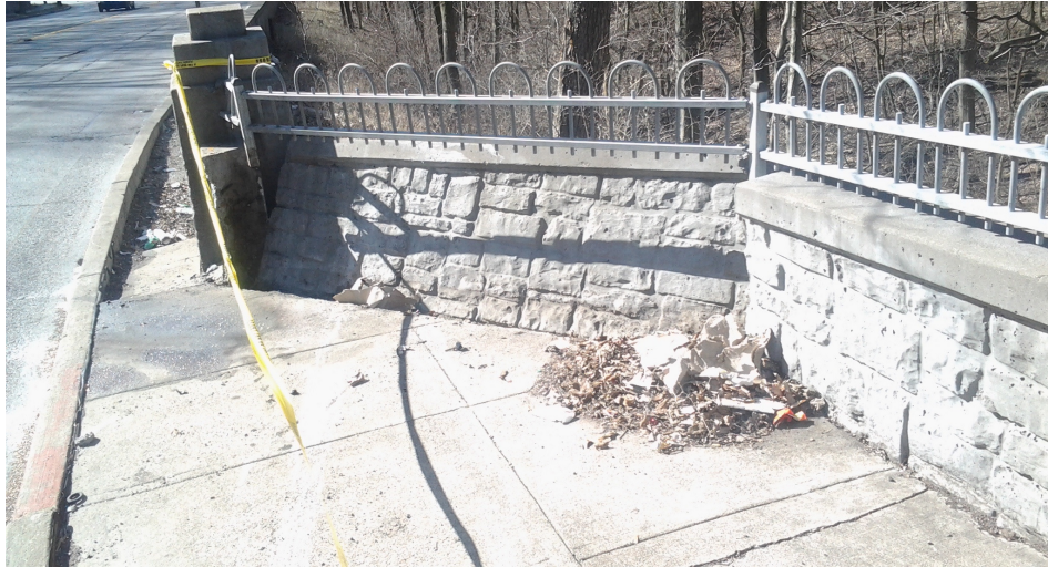
Damaged bus stop opposite Tranquility Lane.
