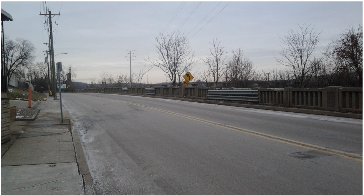
Sections of concrete railing replaced with guardrail sections bolted to pilasters on Cummins Street.
