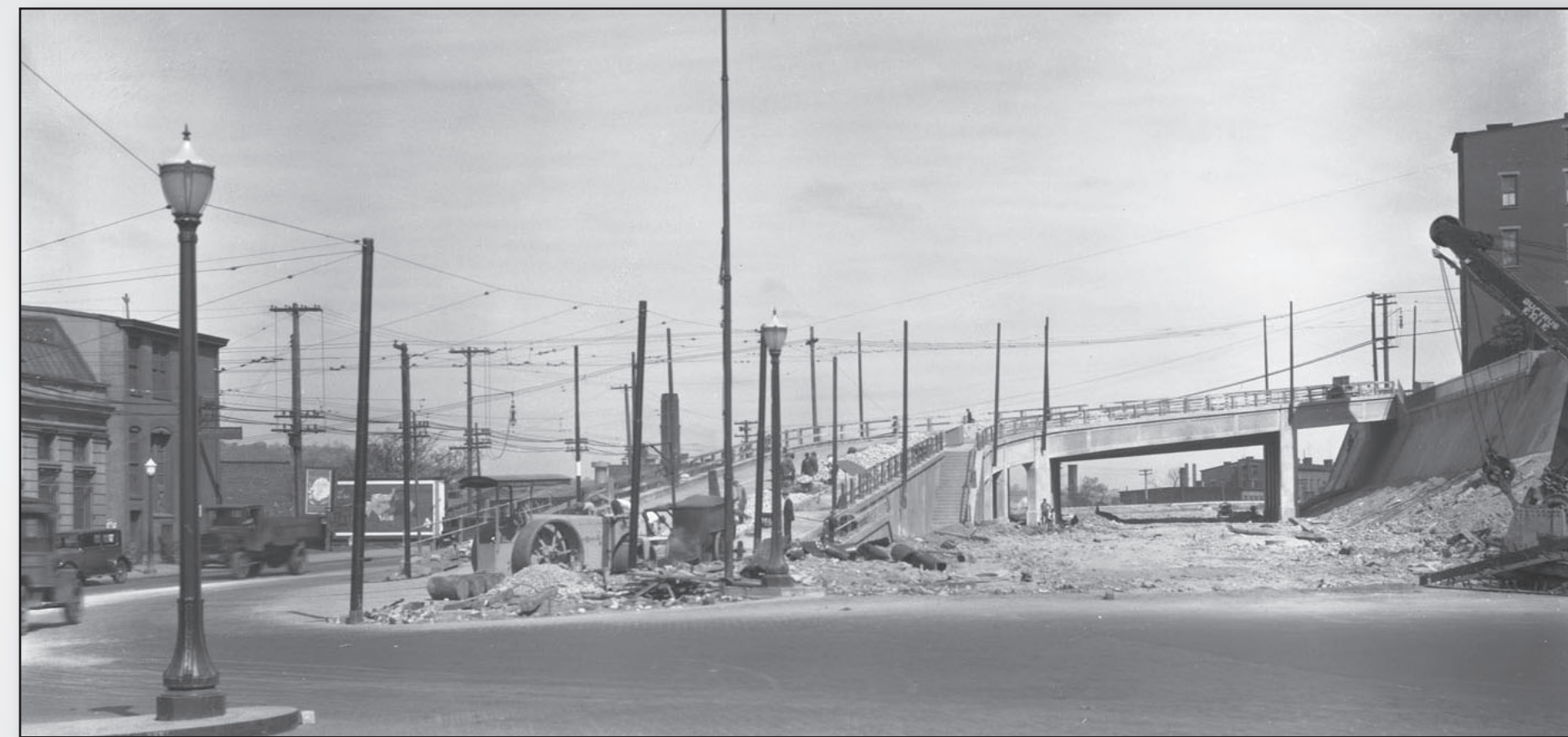
Construction wraps up on the new bridge and the subway that runs below
