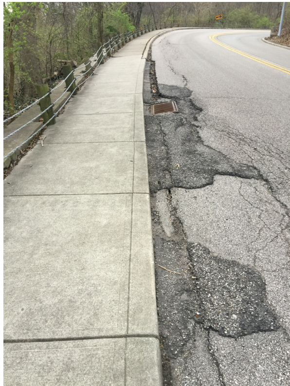
Patchwork to fill gaps due to hillside movement between curb and pavement.
