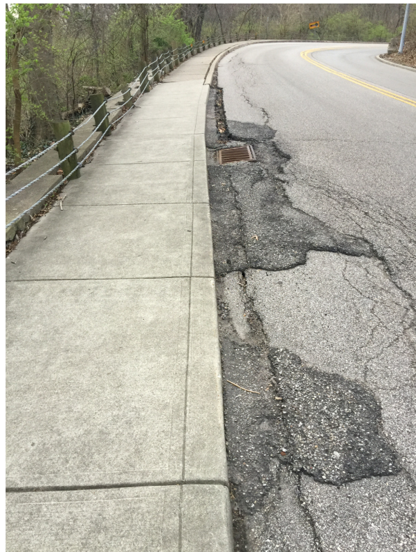
Patchwork to fill gaps due to hillside movement between curb and pavement.
